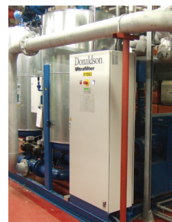
Newly installed air dryers
